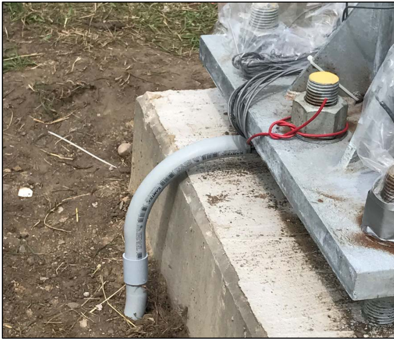
Figure 3.9 - Conduit Leading to Data Logger
