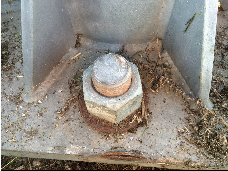
Figure 1.31 - Rusted Washers Found in District 6
