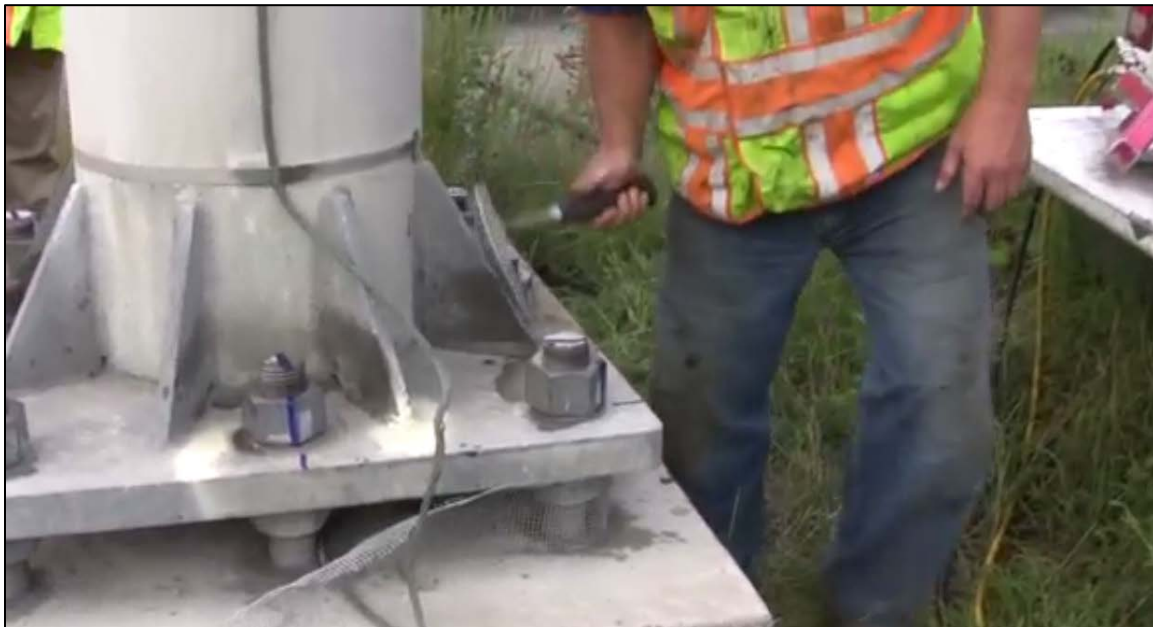
Figure 1.18 - Washers Struck to Inspect Nut Tightness
