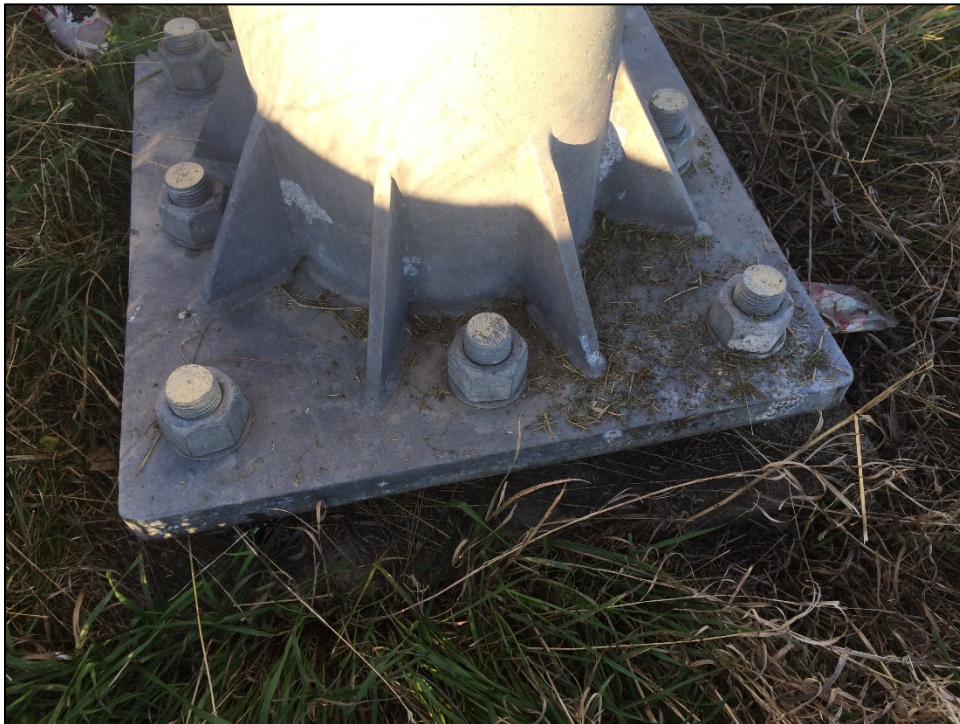
Figure 1.32 - Undersized Washers Found in District 6
