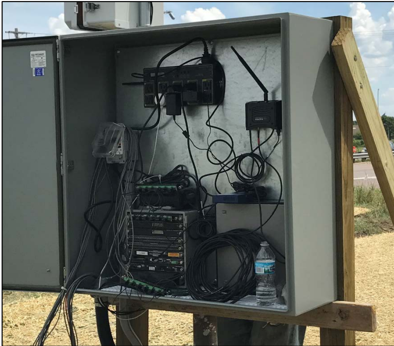
Figure 3.11 - View of Interior of Cabinet
